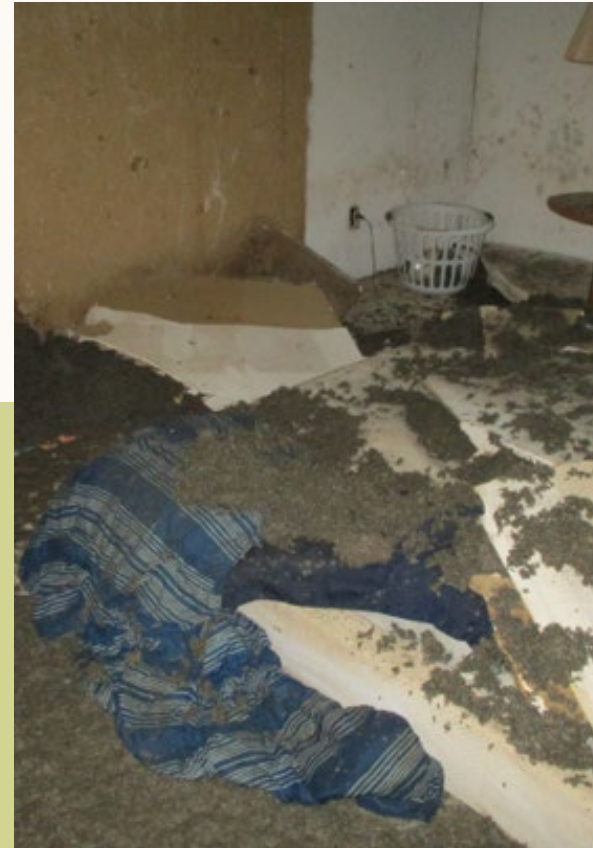
DEBRIS FROM CEILING DAMAGE; WATER DAMAGE AT WINDOW AND WALL
