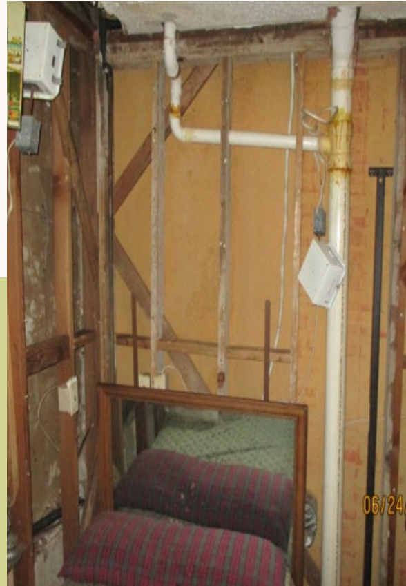
EXPOSED ELECTRICAL WIRING; EXPOSED PLUMBING; MISSING INTERIOR WALLS
