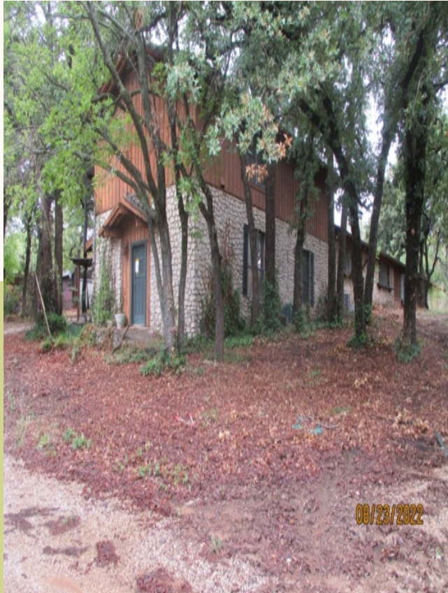
SUBSTANDARD RESIDENTIAL STRUCTURE
