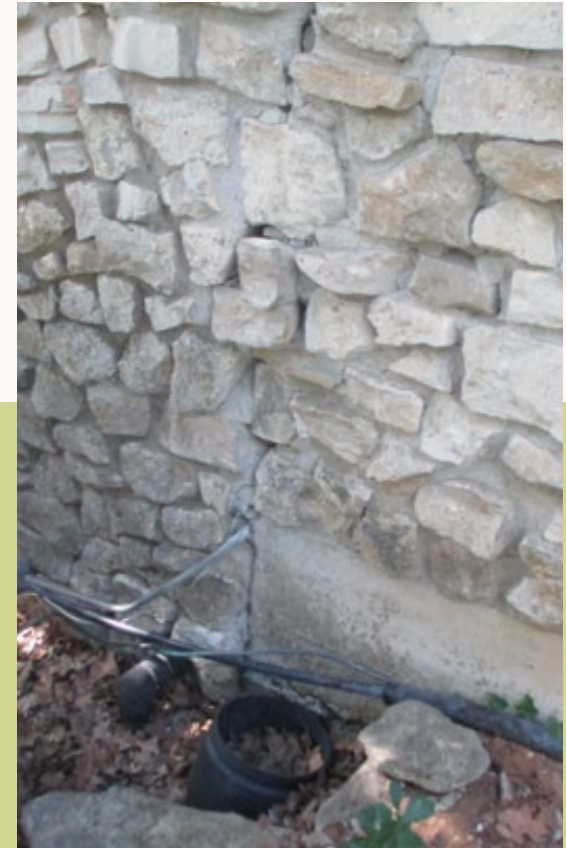
EXTERIOR WALL CRACKS
