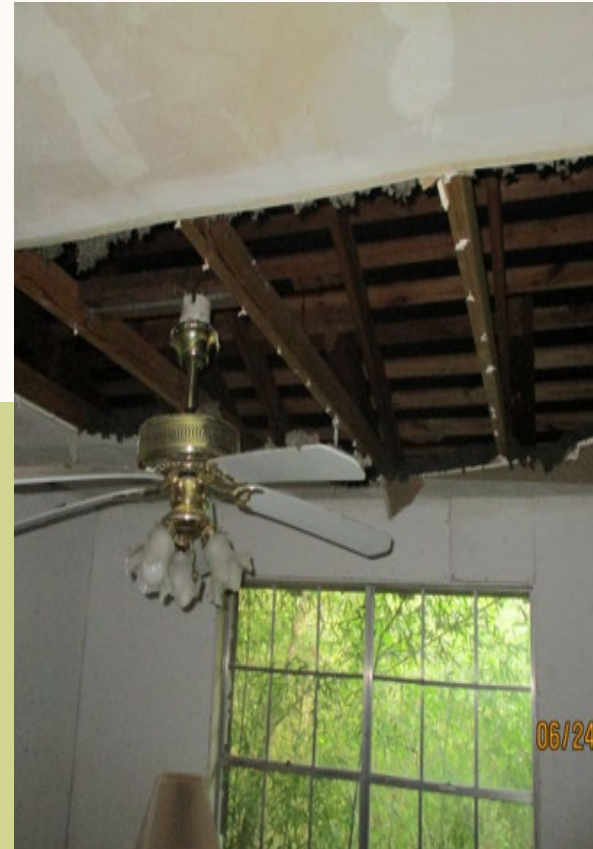
DAMAGED SHEET ROCK IN CEILING
