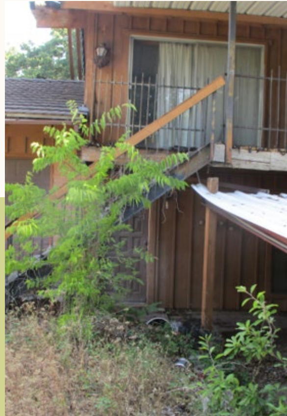
CARPORT DETACHED FROM THE 2 ND STORY; STRUCTURAL HAZARD
