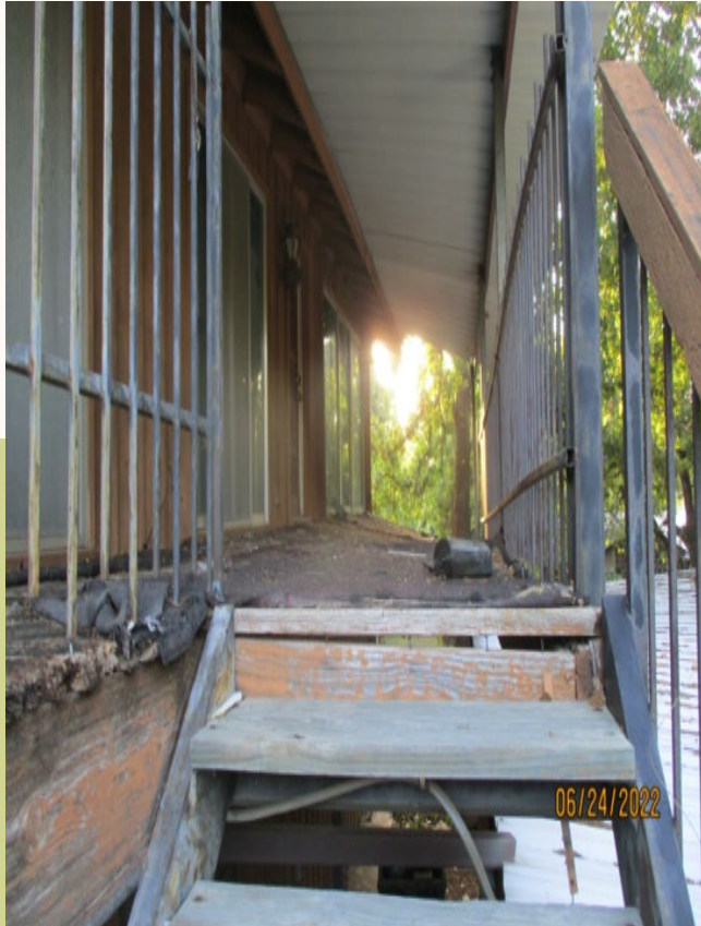
ROTTEN BROKEN WOOD ON 2 ND FLOOR DECKING; 50% OF RAILING MISSING
