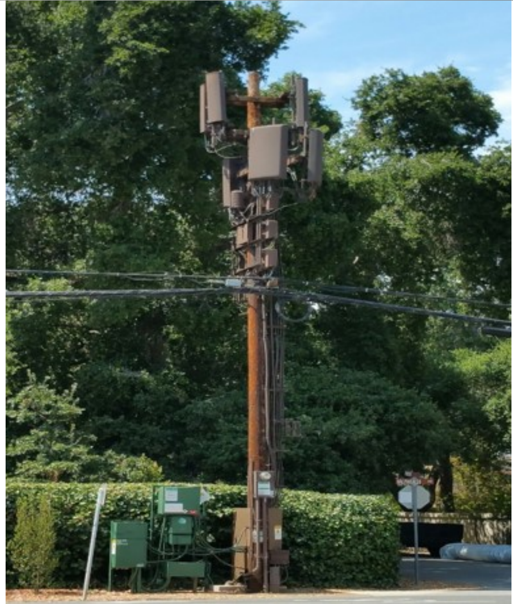
Example of a cluttered small cell install
